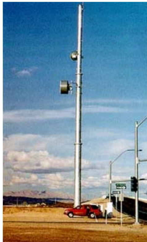
Monopole used in Clark County
